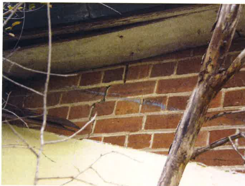
Photo No. 8: 10mm crack at eaves.
