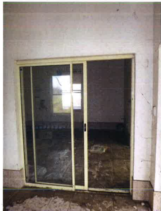
Fig. 31 Original doors have been deleted and unsympathetically replaced
