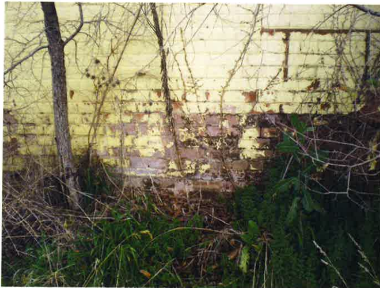
Photo No. 6: Rising damp visible.
