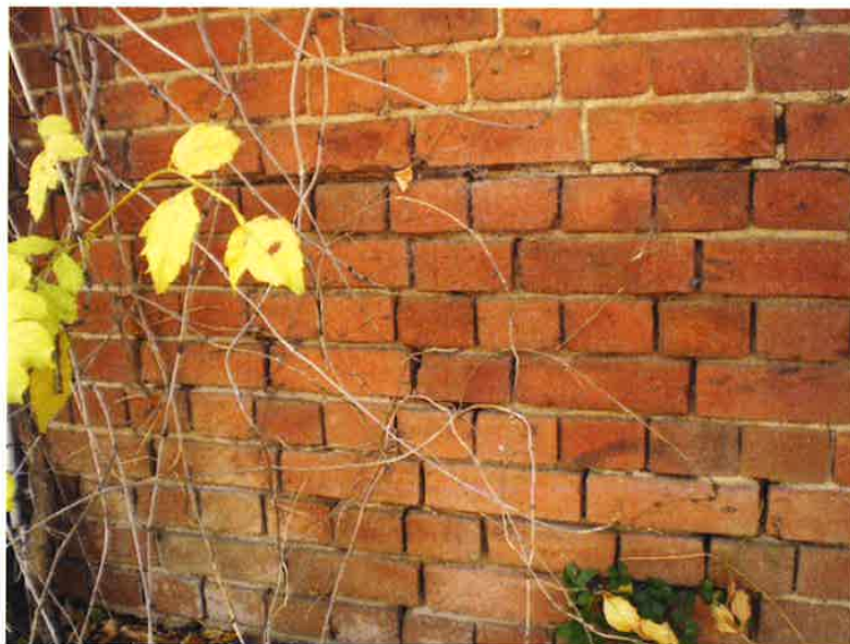
Photo No. 3: Mortar damage – loss of mortar.
