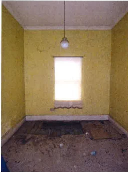
Fig.3 Rear room on south east corner, The floor has collapsed. The floor is covered by animal droppings. Cracking is apparent in all walls.
