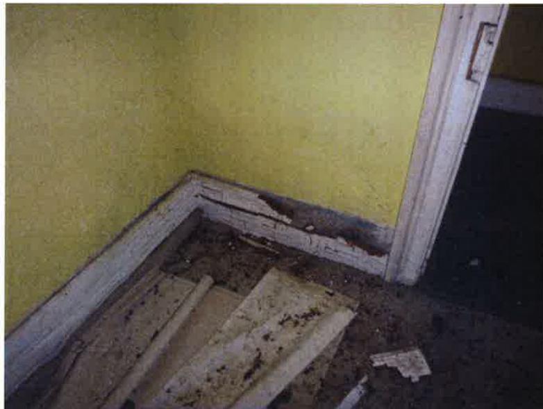
Fig. 16 The skirting has rotted and has been removed from some sections.
