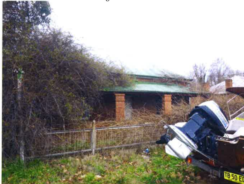
Fig. 22 Veranda, Street façade The fence is not original and the garden is overgrown and has penetrated the roof cavity.
