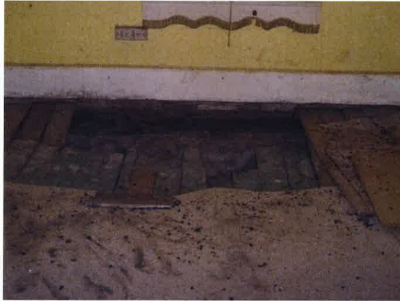
Fig. 7 Collapsed section of the floor.
