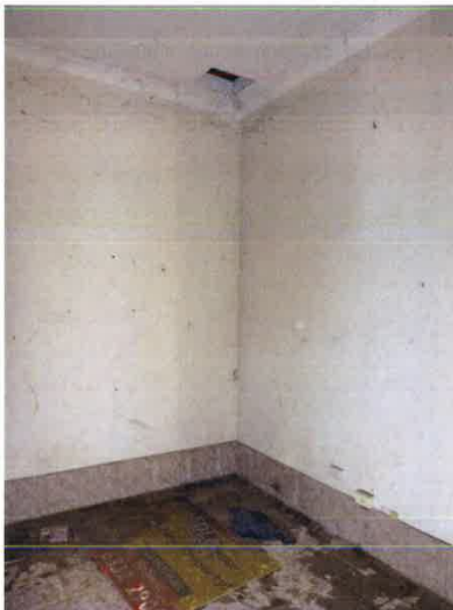
Fig. 30 The building has flooded
