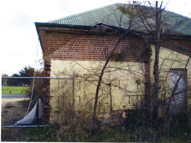
Photo No. 5: Poor workmanship to demolished rear section water free to enter roof cavity.
