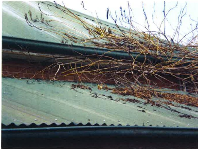
Photo No. 2: Eaves damage, plant ingress.
