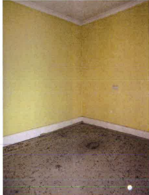
Fig. 11 Animal droppings on the floor of the front (south west room)
