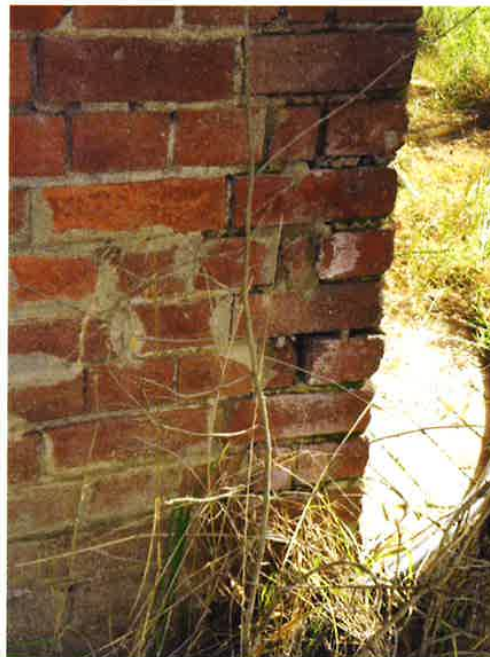
Photo No. 10: Loose bricks and mortar damage
