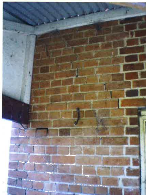
Photo No. 12: 8mm stepped cracking.
