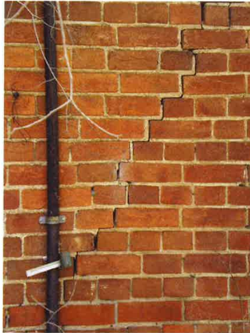
Photo No. 9: 5-8mm vertical crack
