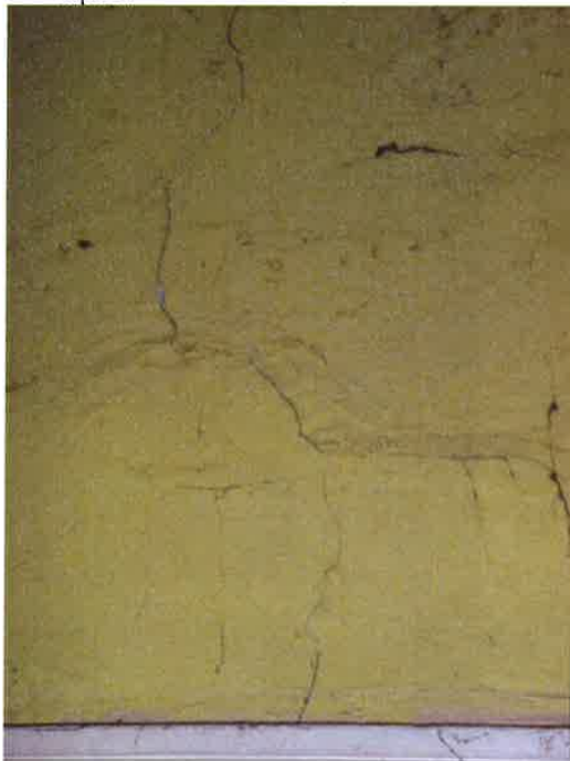
Fig. 8 Hallway (walls are in very poor condition.)
