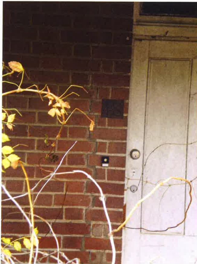
Photo No. 1: Previous repair to crack.
