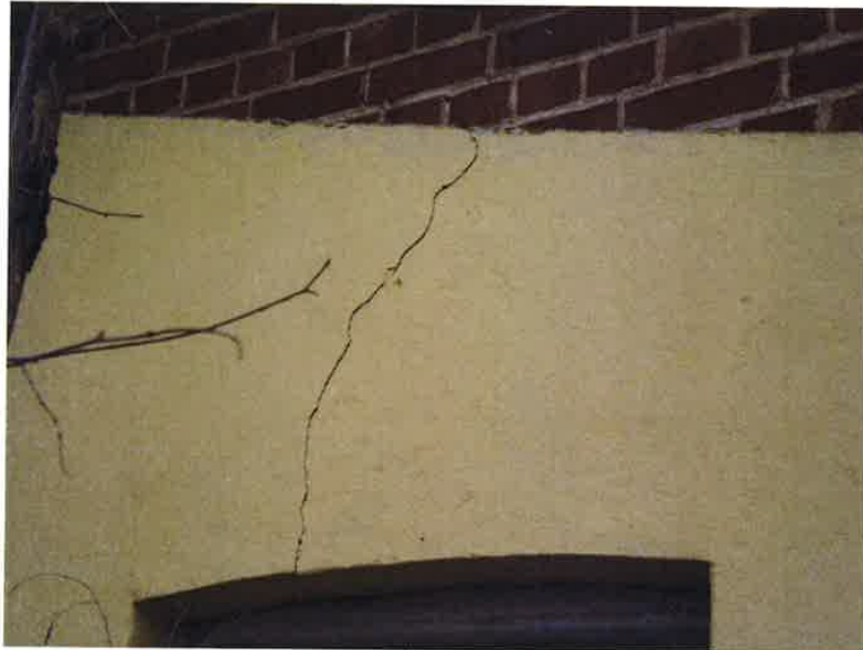
Photo No. 7: 3mm crack above door head.
