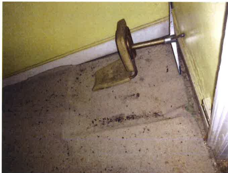
Fig. 4 Section of collapsed floor in rear room.
