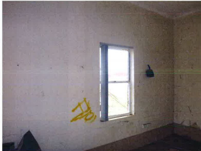
Fig. 29 This section of the house also suffers from dilapidation. Neglect has led to water damage of the walls.
