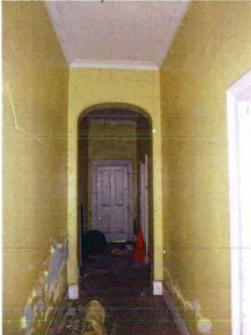
Fig. 10 Hallway is in advanced dilapidated state.
