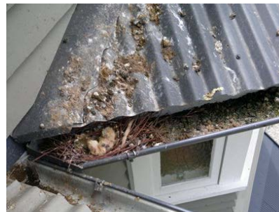
Pigeon nest and droppings on roof
