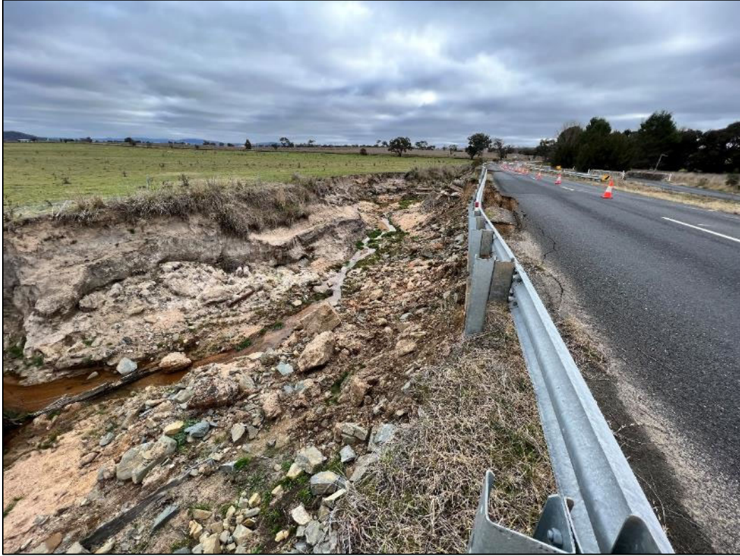
Plate 4: Road and culvert failure along southern side of road verge.
