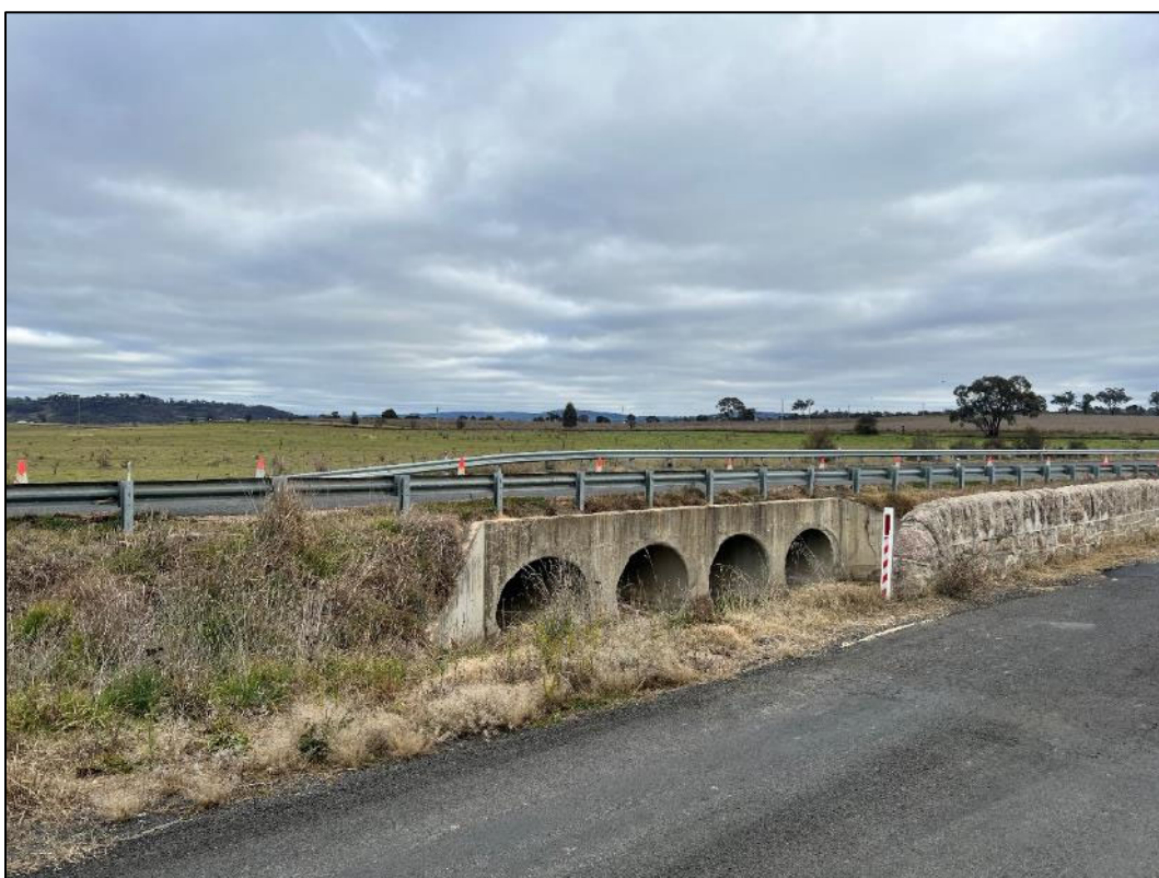
Plate 7: Looking south east across the road failure section from the bypass section to the north.
