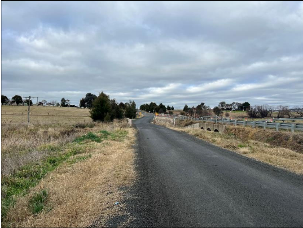
Plate 8: Looking east along the bypass section north of the road/culvert failure along Freemantle Road.
