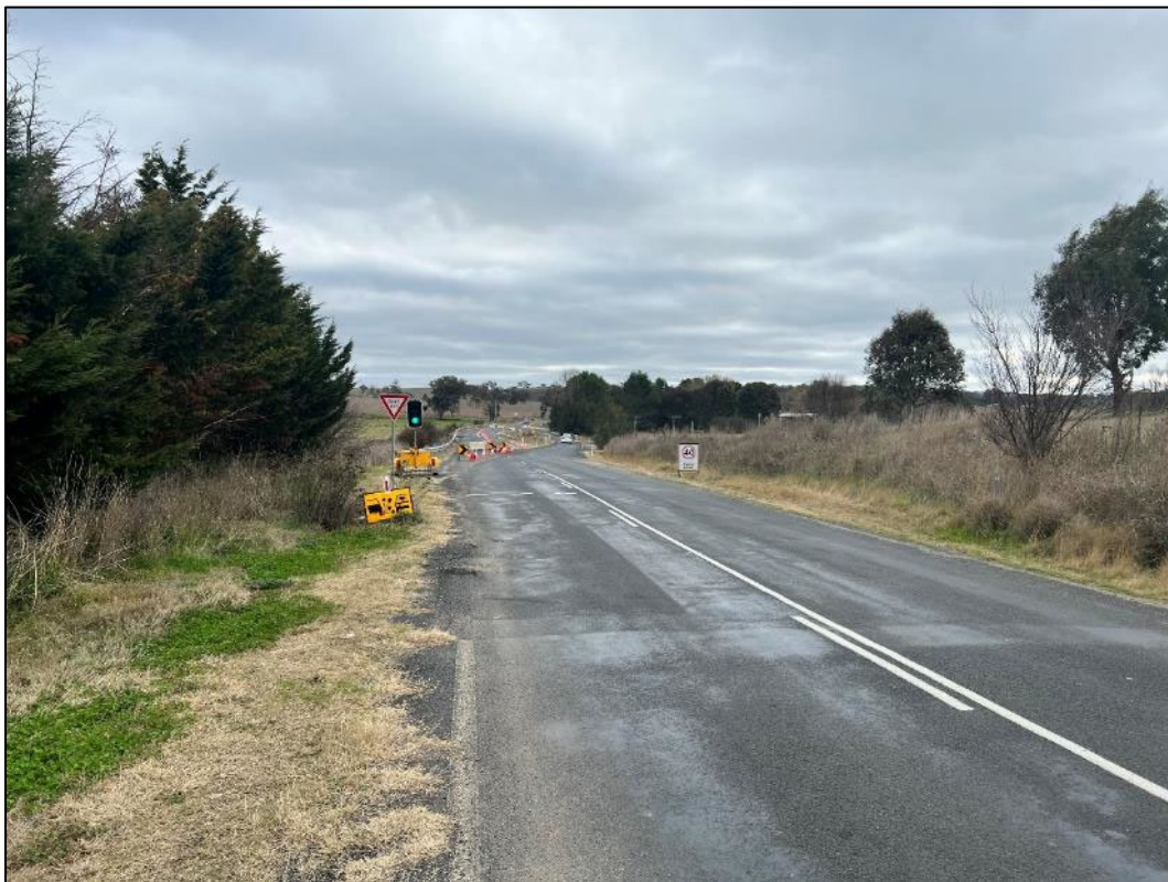
Plate 1: General view looking west from the eastern end of the repair section along Freemantle Road.
