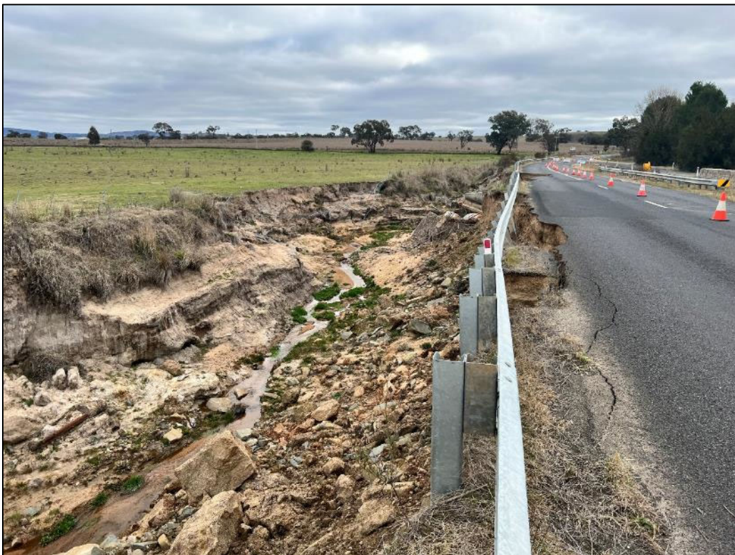
Plate 3: Road and culvert failure along southern side of road verge.
