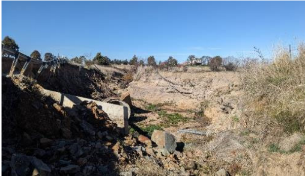
Plate 1 Eroded creek banks and creek bed containing rubble within the subject site
