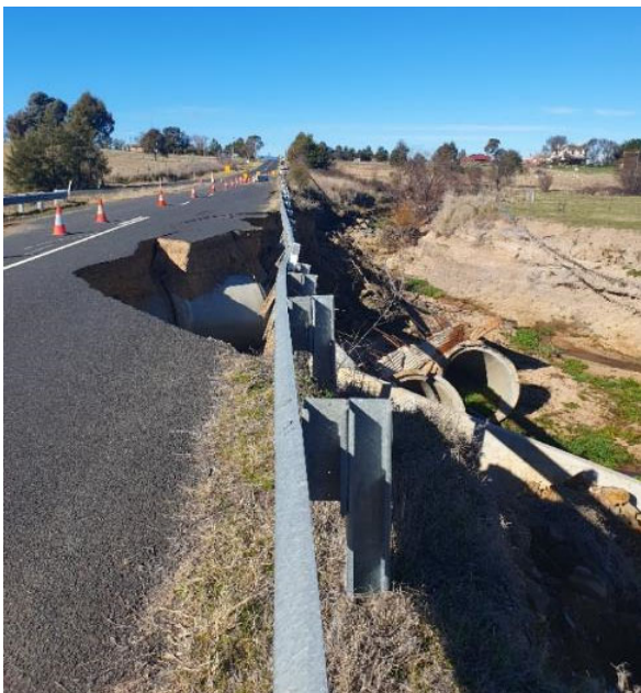
Plate 23 Collapsed culvert and road edge along southern section of Freemantle Road
