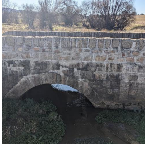
Plate 6 Pooling water between Kelloshiel Creek Stone Bridge and the culvert
