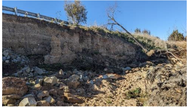
Plate 2 Eroded creek bank along the southern edge of Freemantle Road
