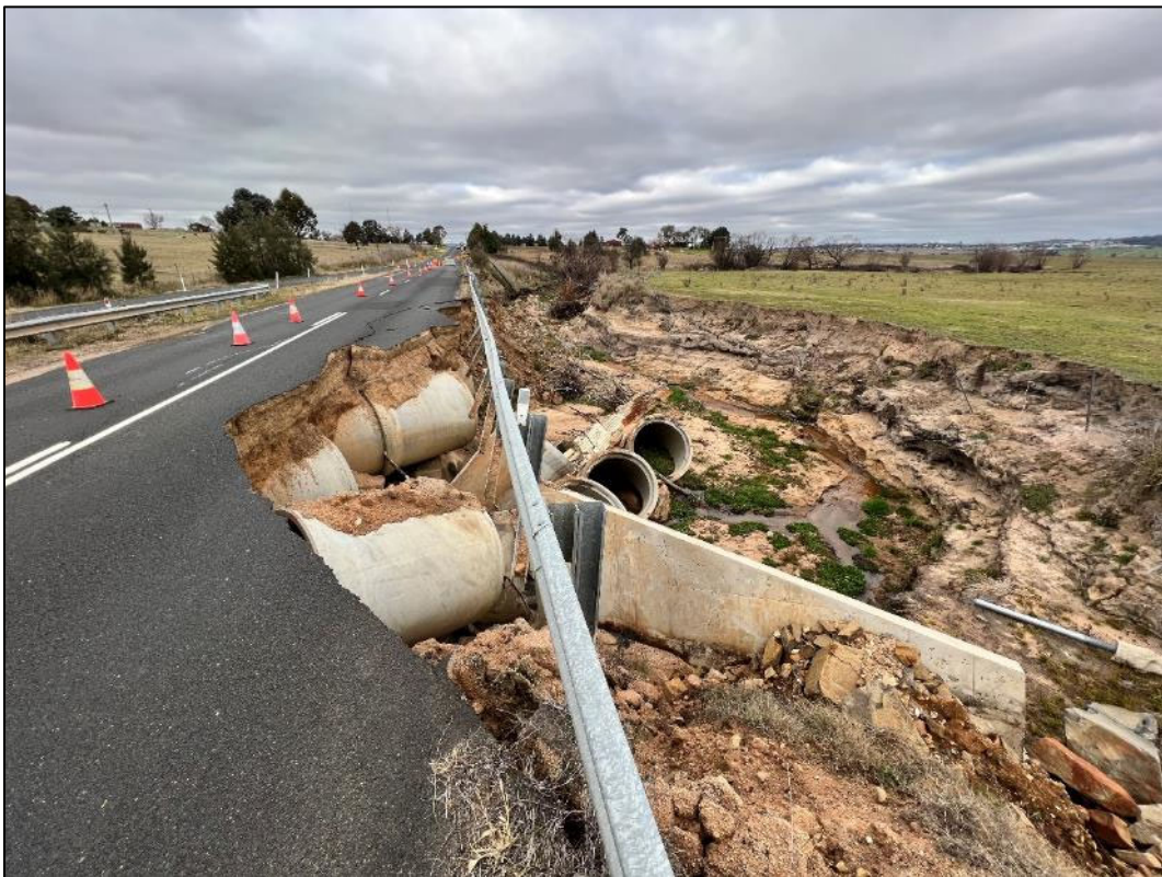
Plate 5: Road and culvert failure along southern side of road verge looking east.
