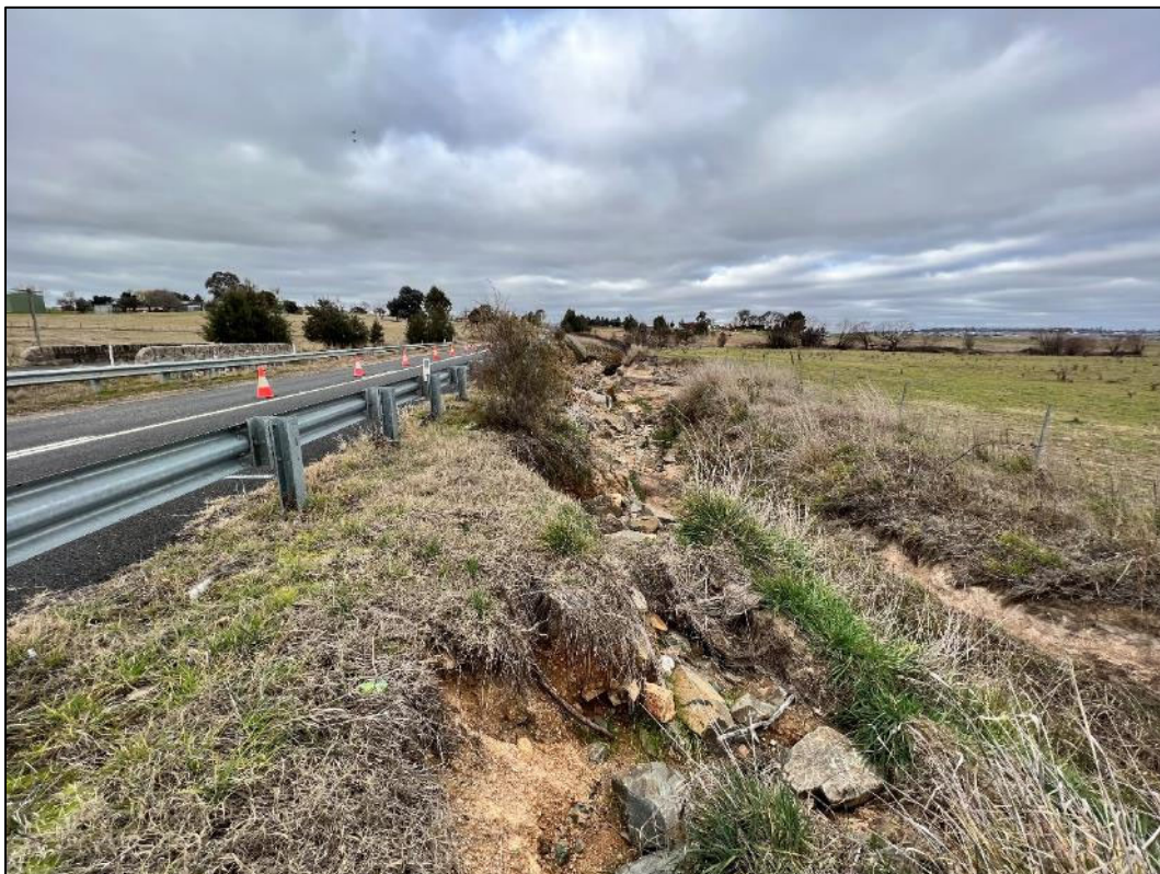
Plate 6: Looking east from the western end of the road failure section along Freemantle Road.
