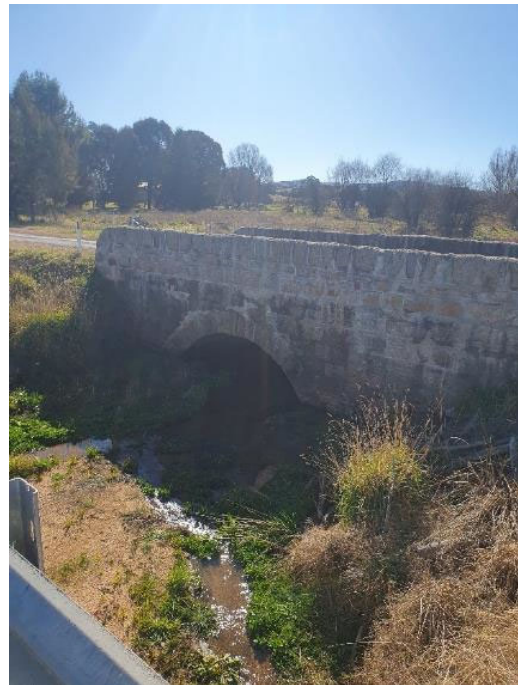
Plate 16 Pooling water within Kelloshiel Creek. Site of the temporary dry work holding pool.
