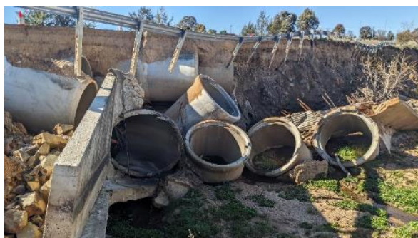
Plate 17 Collapsed Freemantle Road Kellosiel Creek culvert
