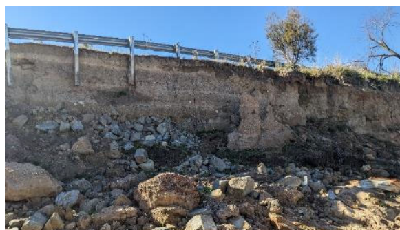
Plate 18 Under cut and eroded southern road edge
