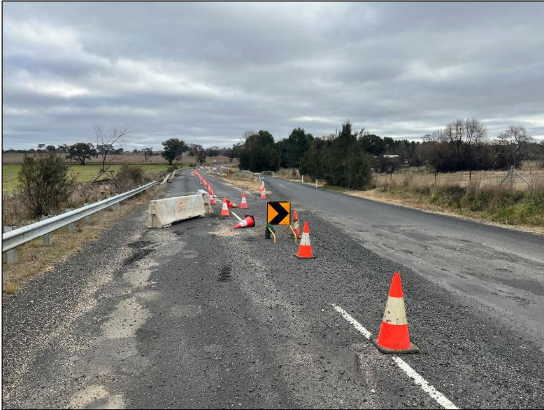
Plate 2: Looking west along the repair section of Freemantle Road. Start of road failure along the southern side of the road.
