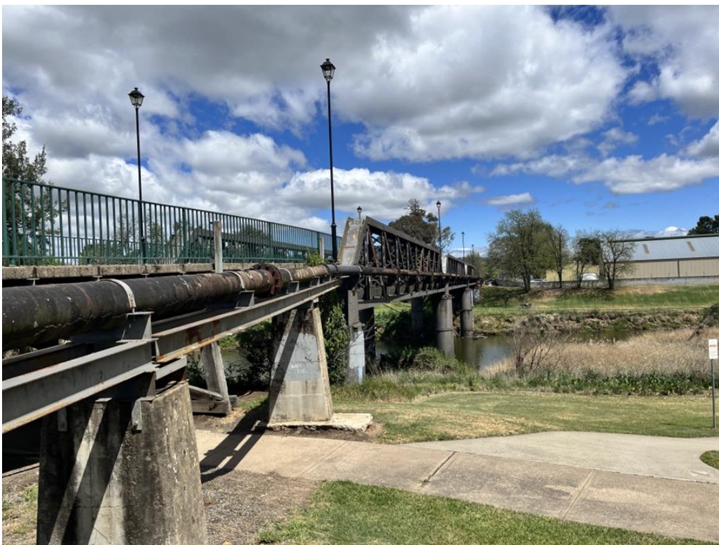
Figure 33. Denison Bridge from eastern bank looking towards western bank, showing existing water main affixed to downstream side of bridge. Vertical section of proposed pipeline will be attached to the downstream side of the second pylon in the foreground of the photograph. Source: Premise.
