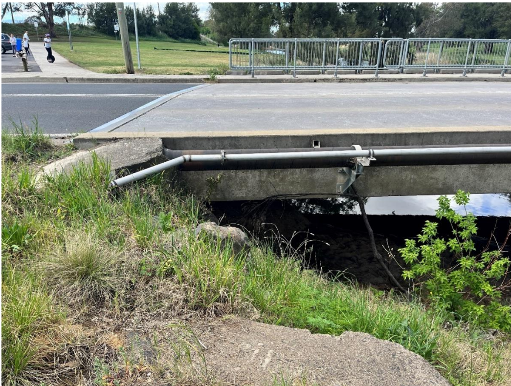
Figure 35. Hereford Street Bridge looking at eastern bank, downstream side of bridge. Source: Premise.
