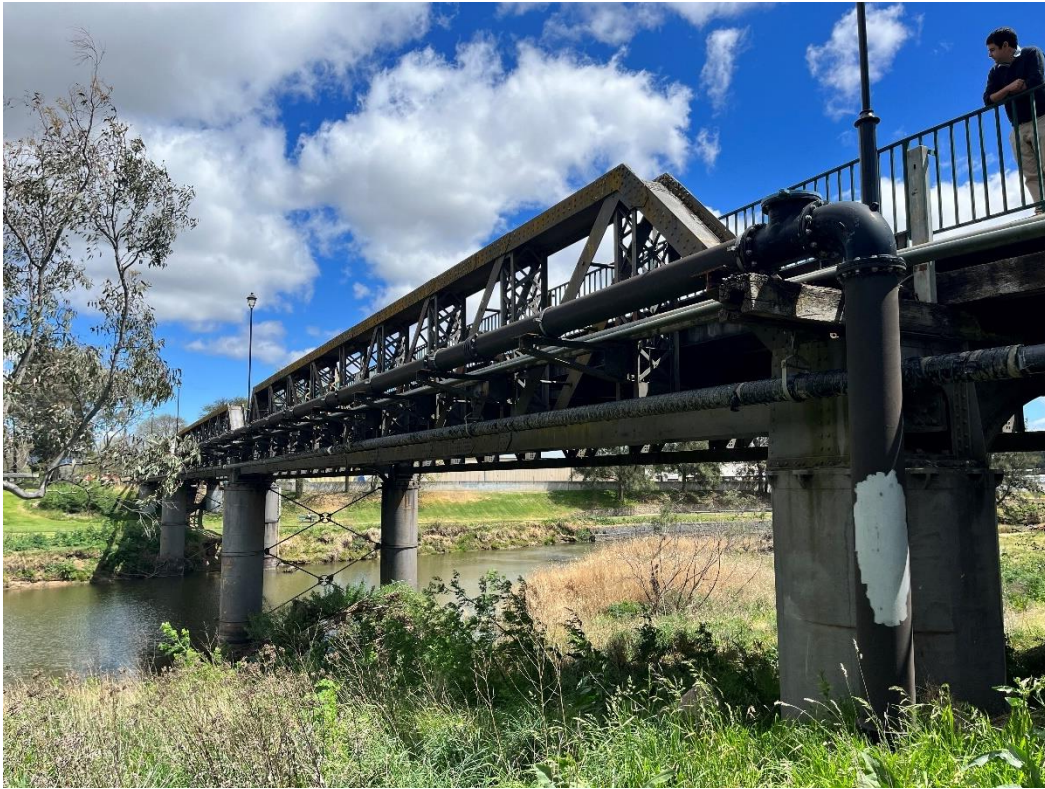
Figure 32. Denison Bridge from western bank looking towards eastern bank, where existing water main emerges from ground to bridge, downstream side of bridge. Source: Premise.
