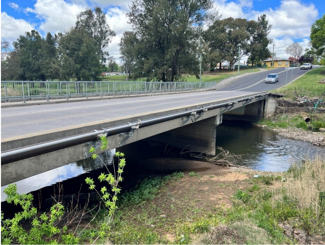
Figure 34. Hereford Street Bridge from eastern bank looking towards western bank, downstream side of bridge. Source: Premise.
